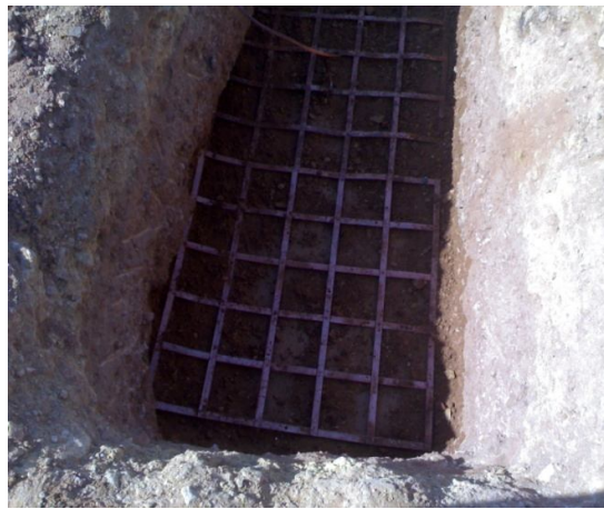
Fig. 13 Photograph of the earthing pit with grounding mesh
