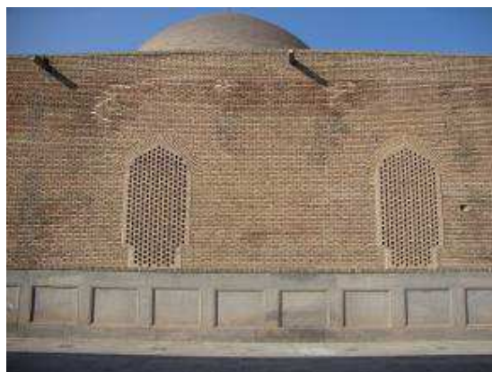
Fig. 11: a sample of meshy walls at the opposite of openings at eastern and western frontage [11]
