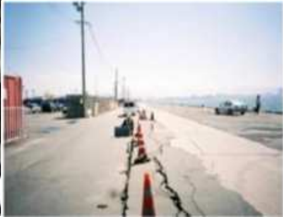
Fig.5. Damage to the wharf
