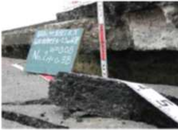
Fig.4.Ground settlement in liquefaction
