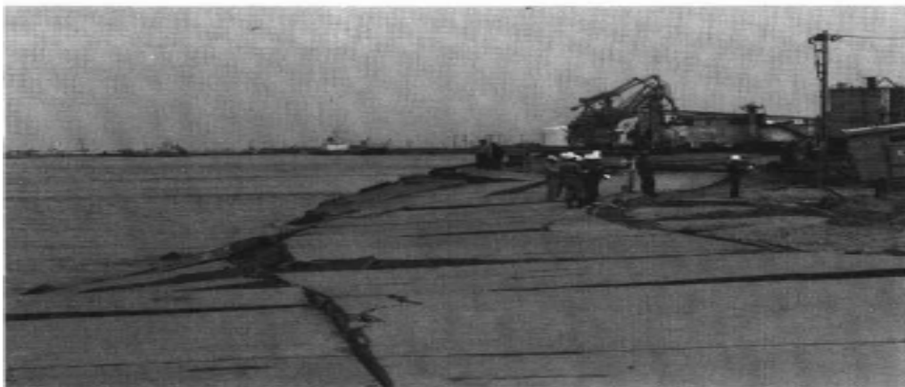
Fig.1. Damage to a sheet pile quay wall at Shimohama Wharf, Akita Port, Japan, during the Nihonkai-chubu earthquake of 1983.
