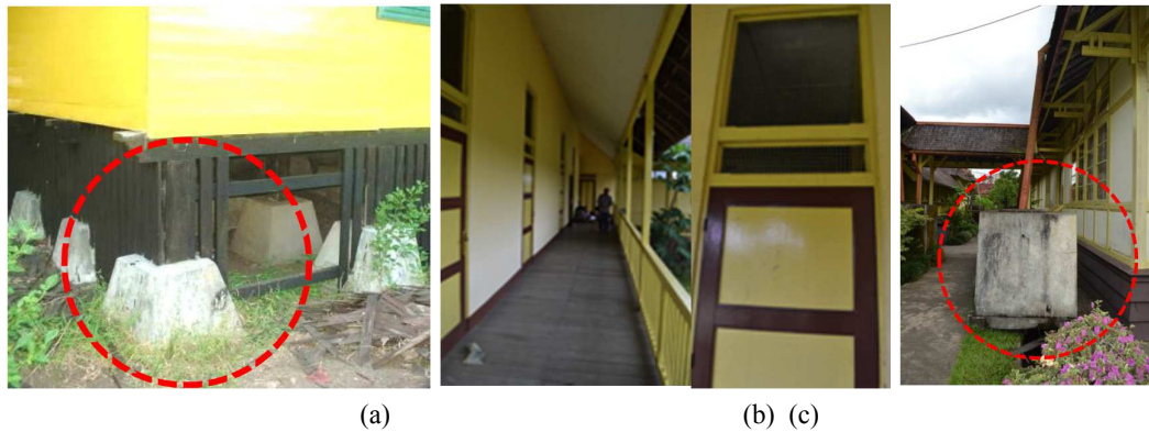
Figure 9. (a) Pedestals Foundation, (b) Large Doors and Windows, (c) Water Reservoir Source: Field Survey, 2012
